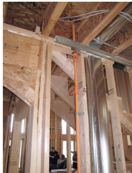
BlazeMaster pipe was installed in a Kenosha firefighters new home last spring.
